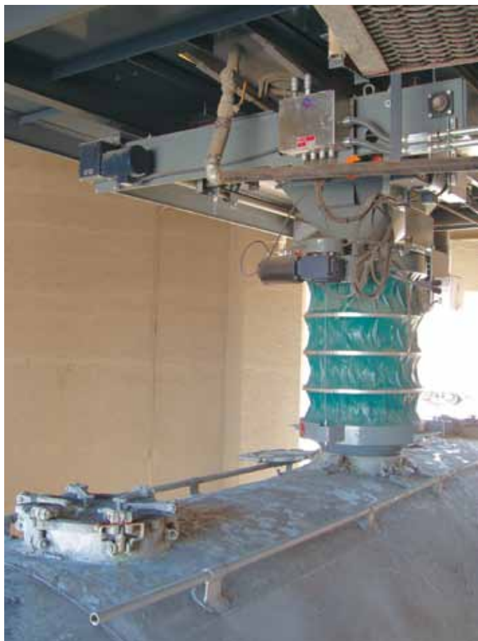
Heavy duty application: DCL load spout loading cement
